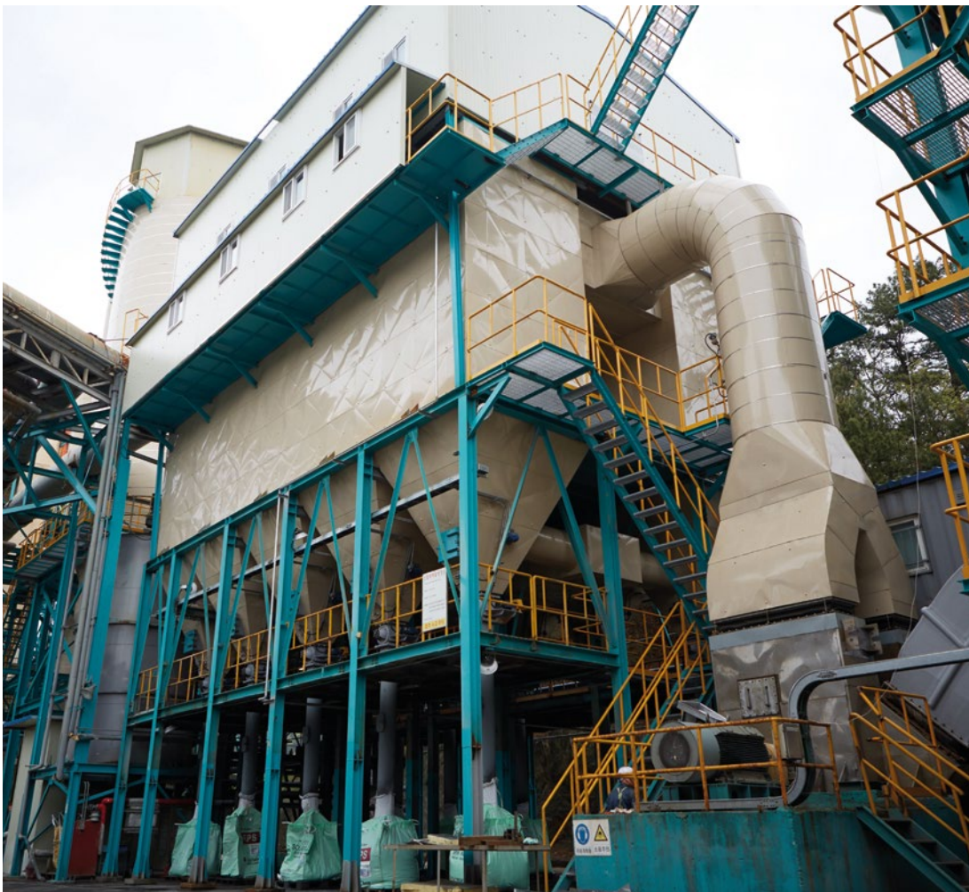
EMK operates six WTE plants and five sludge drying facilities and has the third largest incineration capacity in South Korea.
