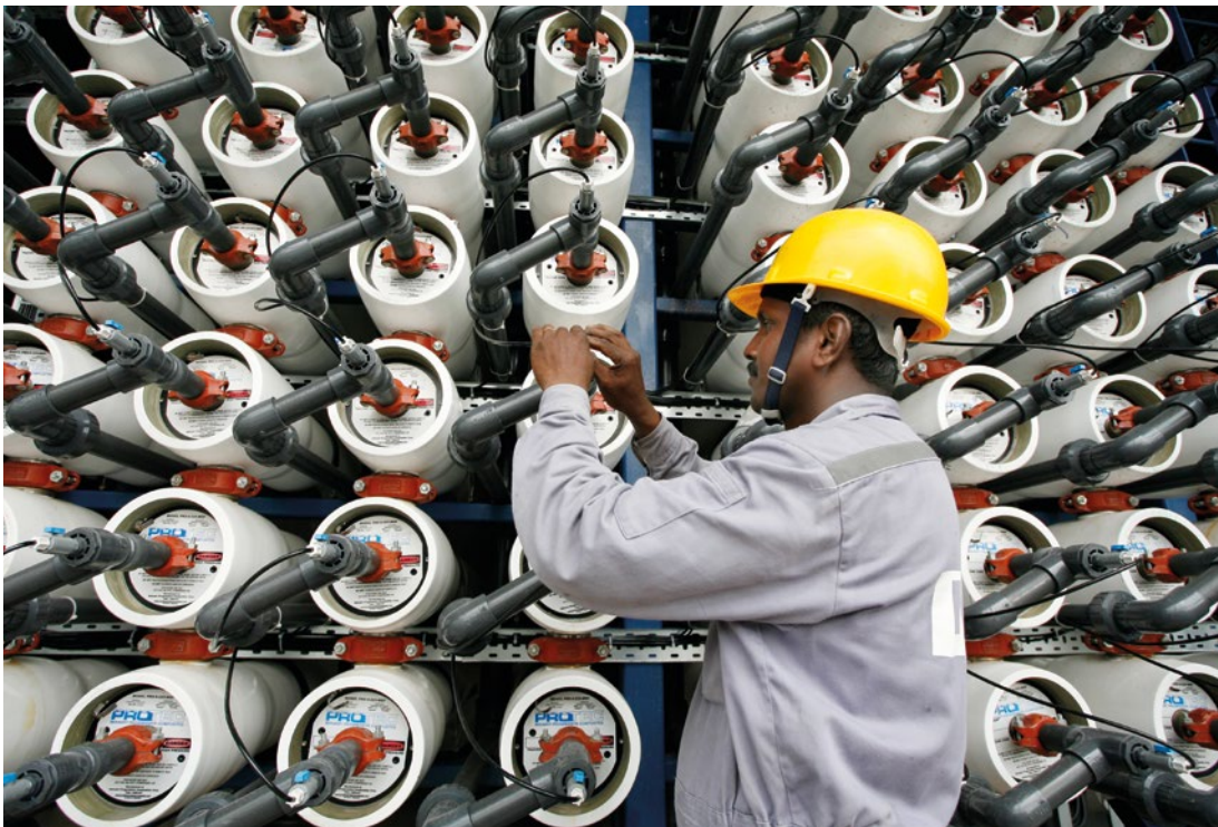
The Keppel Seghers Ulu Pandan NEWater Plant achieved 100% plant availability in 2022.
