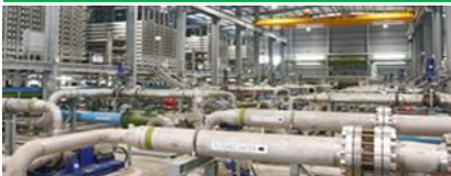
SingSpring Desalination Plant
