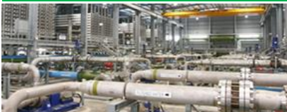
SingSpring Desalination Plant
