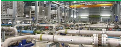
SingSpring Desalination Plant
