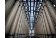
Keppel Seghers Ulu Pandan NEWater Plant
