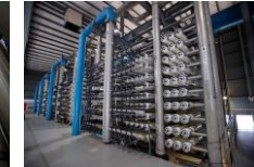
SingSpring Desalination Plant
