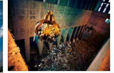
Keppel Seghers Tuas WTE Plant
