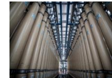
Keppel Seghers Ulu Pandan NEWater Plant
