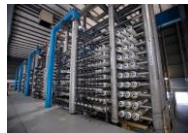
SingSpring Desalination Plant
