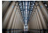
Keppel Seghers Ulu Pandan NEWater Plant
