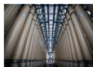
Keppel Seghers Ulu Pandan NEWater Plant
