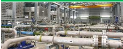
SingSpring Desalination Plant
