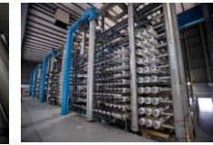
SingSpring Desalination Plant
