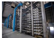
SingSpring Desalination Plant
