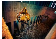
Keppel Seghers Tuas WTE Plant
