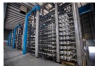
SingSpring Desalination Plant
